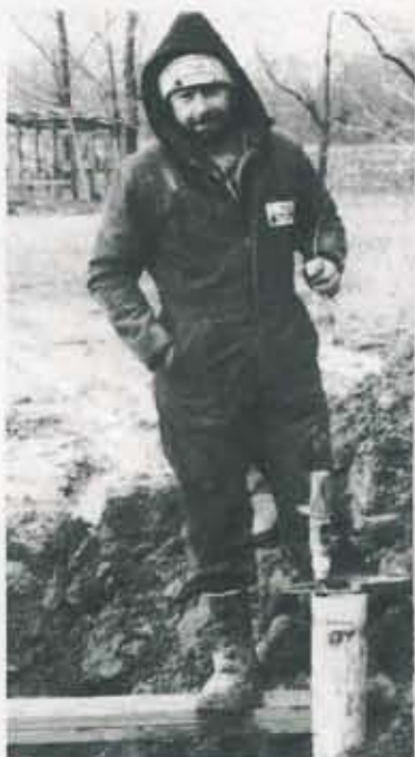
A GENESIS INSTALLER begins making the connections that will tie the cased closed loop into the heat pump itself.
