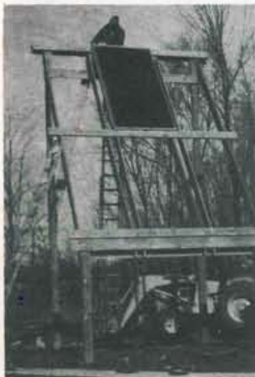
GENESIS ENERGY SYSTEMS not only installed the collectors for the system in Avilla, Ind., it also built the rack they sit on. The collectors are used to heat the swimming pool in the summer and the cased storage-heat exchanger tube in the winter, as well as to provide domestic hot water.
