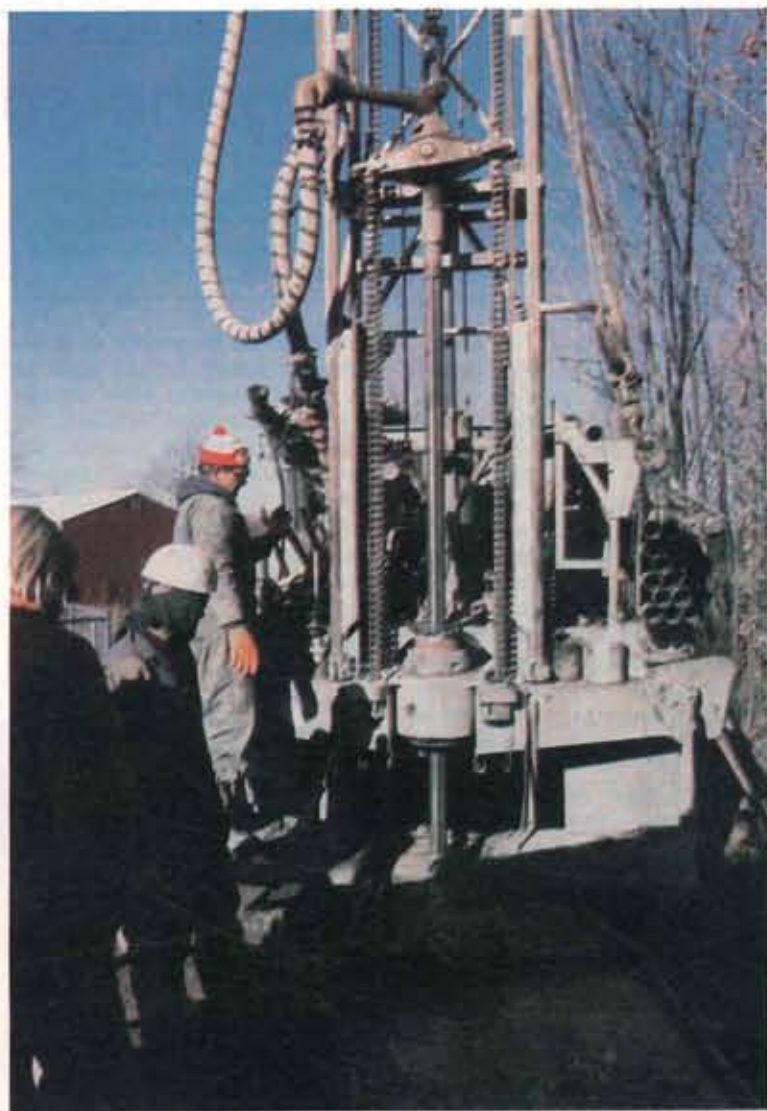
FOR VERTICAL PLACEMENT of the closed loop, a hole is dug with an ordinary drilling rig. The plastic or steel casing is then inserted, with the polybutylene piping making a loop within the casing. The casing is then capped, or pressurized. At this installation in Avilla, Ind., the loop was installed 320 ft deep.
