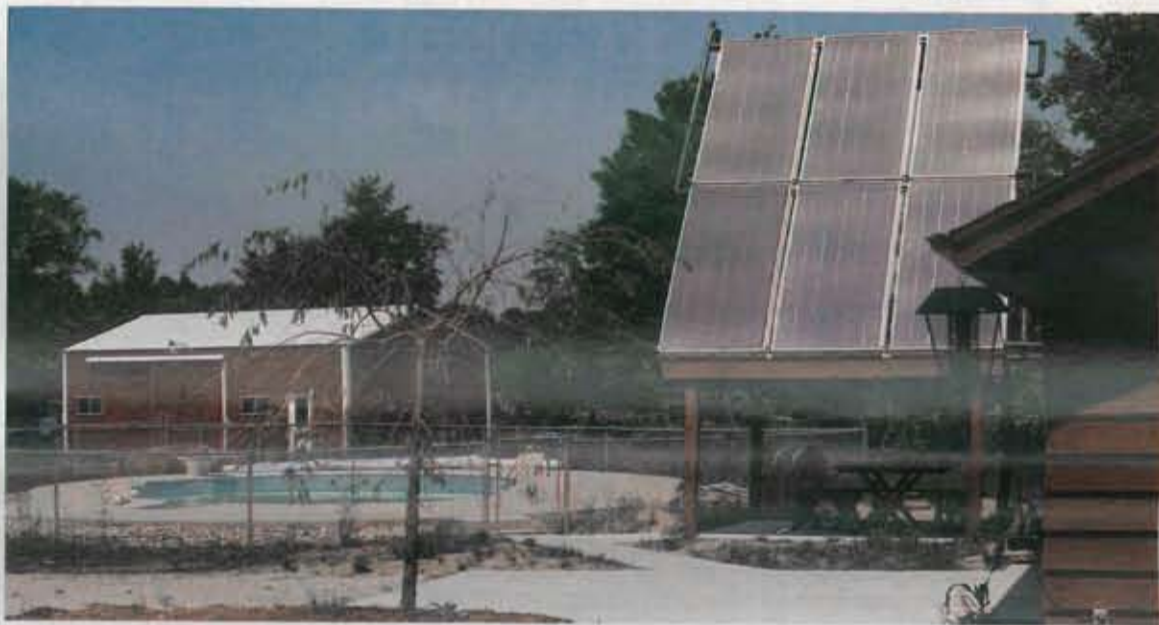
GENESIS ENERGY SYSTEMS, Division of A. Hattersley & Sons, Inc., Fort Wayne, Ind., installed one of its solar assisted, earth coupled, closed loop heat pump systems at this home in Avilla, Ind., in the fall of 1980. The sealed casing containing the closed loop was installed vertically 320 feet deep. The six 4-ft by 8-ft solar collectors heat the swimming pool in the summer and the cased storage-heat exchanger tube in the winter. Heating, cooling, and domestic hot water are provided by a 3-ton Command-Aire heat pump tied to the solar assisted closed loop.
