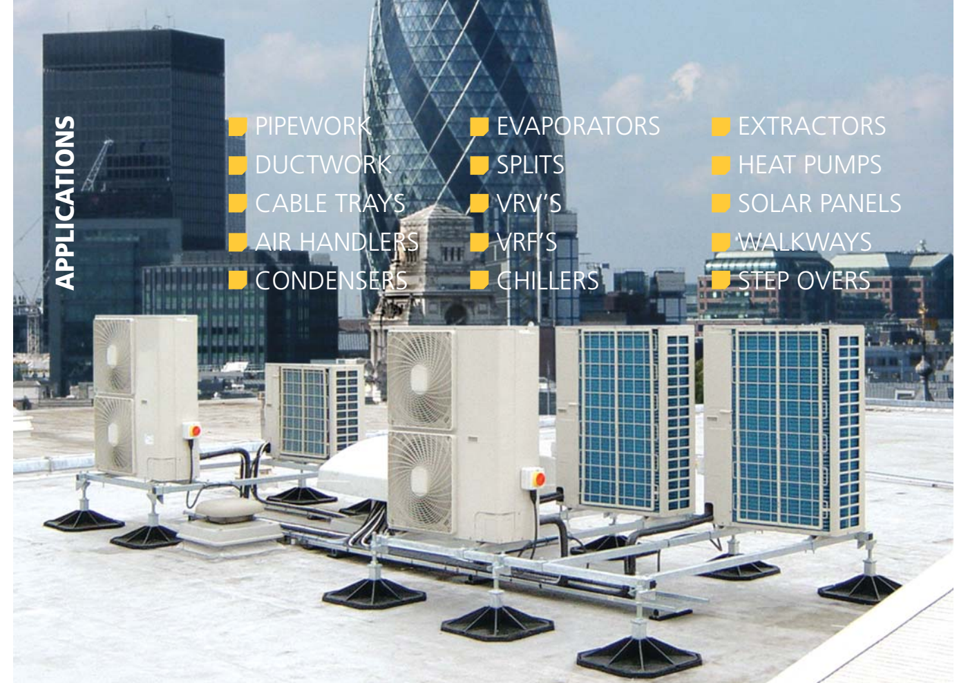
INSTALLED BY SBH DESIGN & INSTALLATION SERVICES LTD
